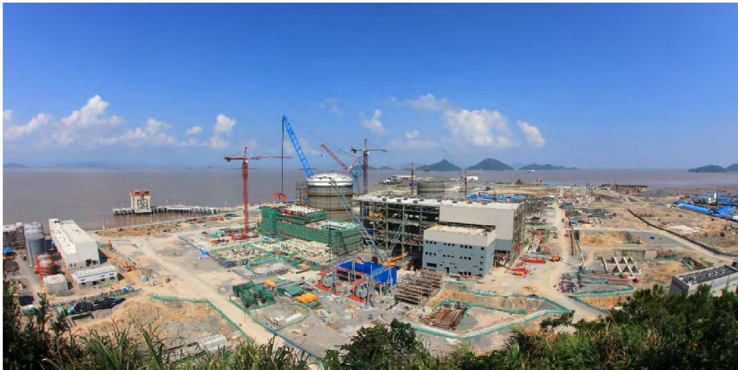
Figure 1 – Sanmen Nuclear Power Plant using AP1000 technology
