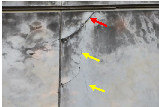
Figure 6. Failed joint filler at a previous repair (red arrow) and cracks (yellow arrows) at a Rock Creek Parkway overhang marble panel (photo taken at the west facade). Note: No existing through-pin visible at the repaired corner stone fragment, potential incipient spall location.
