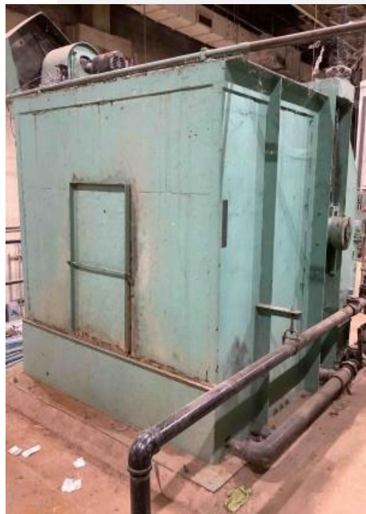
Figure 70. Existing Traveling Screen Unit in Condenser Water River Pump Room
