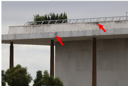
Figure 9. Dark black discoloration at the Plaza Level overhang fascia and coping units (photo taken at the east facade).
