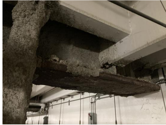
Figure 39. Missing fireproofing at A-level structural support
