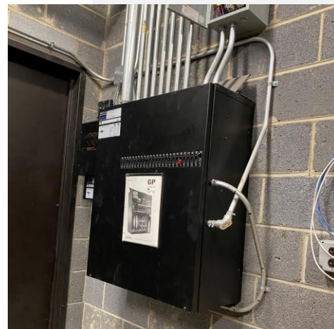
Figure 77. Existing Lighting Control Panel
