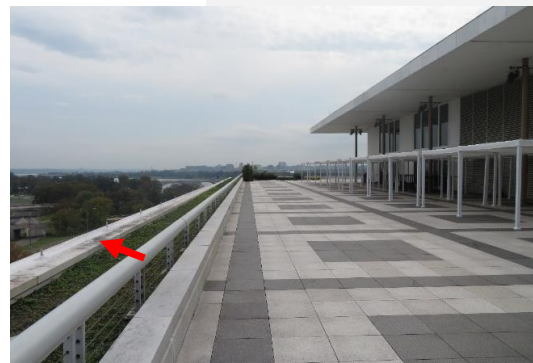
Figure 37. Terrace Level hot-fluid-applied reinforced rubberized asphalt (HRA) membrane and paver assembly roof and marble clad planter. Note the black discoloration on the planter marble coping units (red arrow).
