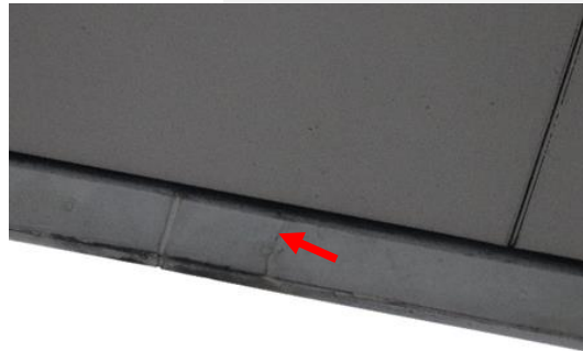
Figure 5. Crack and potential incipient spall location at a Plaza Level overhang marble soffit panel (photo taken at the west facade). Note: The crack aligns with a potential through-pin location; the stone section to the left of the arrow is a potential incipient spall location.
