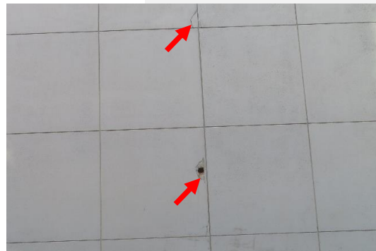
Figure 15. Incipient spall (upper arrow) and spall (lower arrow) coincident with ferrous elements.
