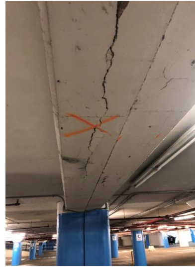
Figure 88. Concrete Cracks at Parking Garage Level C
