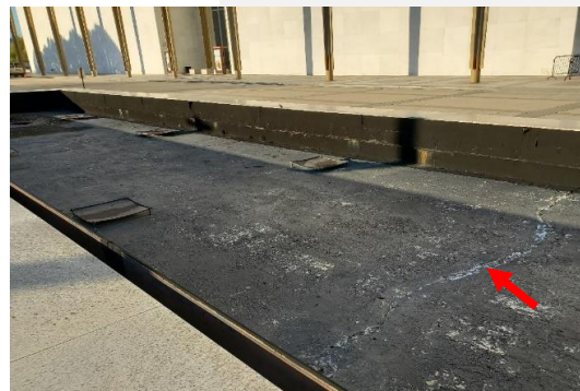
Figure 32. Rectangular reflecting pool basin at the east side of the Plaza Level. Note the crack in the concrete topping that extends through the liner coating.
