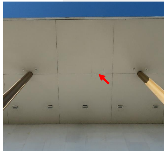
Figure 10. Staining and active leak location at stucco panel joint at the south facade.
