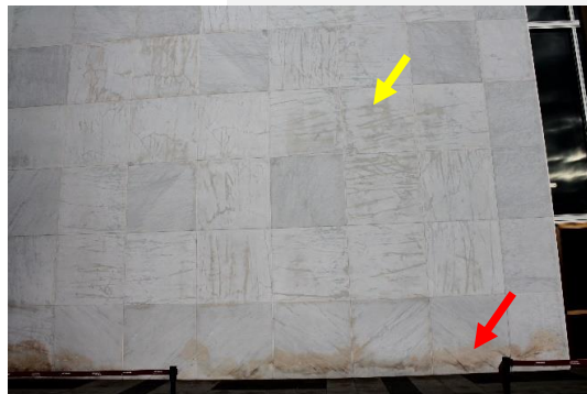
Figure 8. Orange-brown discoloration at the panels along the base of the Plaza Level walls (red arrow) and orange-brown and gray discoloration along veining patterns (yellow arrow) (photo taken at the west facade).
