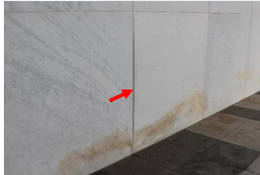
Figure 4. Bowed Plaza Level marble panel (photo taken at the west facade).
