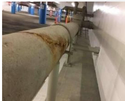
Figure 73. Existing Sanitary Main with Crack
