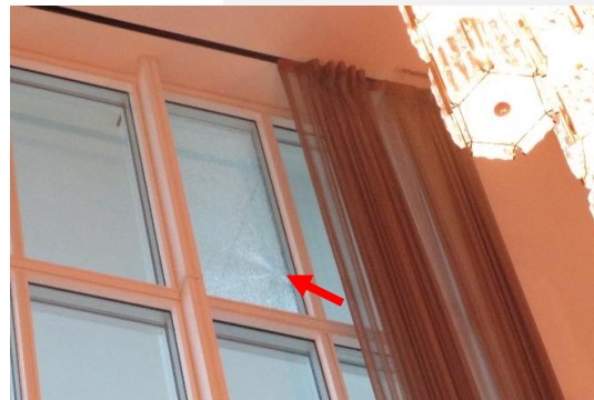
Figure 17. Broken IGU at the Plaza Level west facade.
