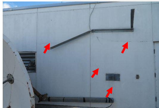
Figure 13. Wider cracks in the stucco adjacent to a previous support for a satellite dish at a Main Roof areaway.
