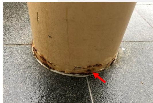
Figure 27. Typical mild corrosion and flaking paint at the base of the Plaza Level columns.
