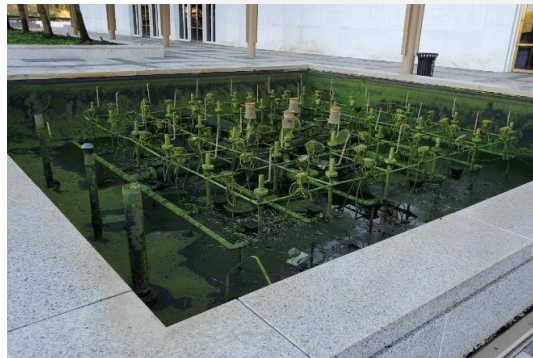
Figure 33. Square fountain at the west side of the Plaza Level with active leaks observed below the pipe penetrations at the Level A parking area below.
