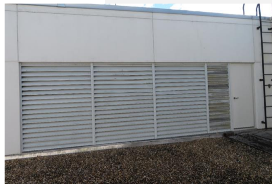
Figure 25. Chalked and missing paint (red arrows) as well as bent blades (yellow arrow) at a Main Roof areaway louver.
