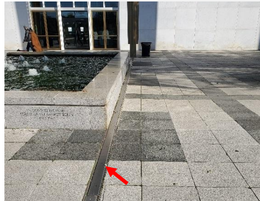
Figure 31. Plaza Level metal expansion joint cover at the west side of the plaza. Note active leaks were observed along this expansion joint at the Level A parking area below.
