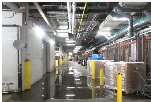
Figure 28. Water collected at the service corridor roadway.
