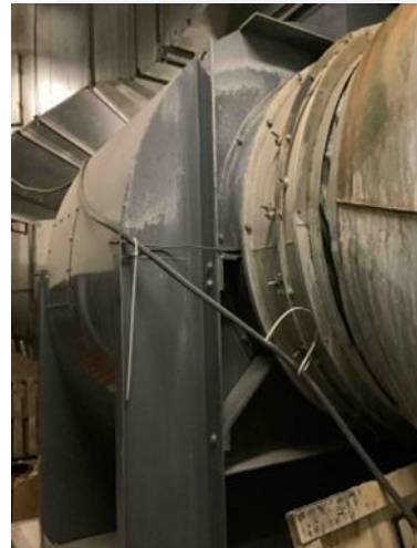
Figure 67. Existing Garage Exhaust Fan
