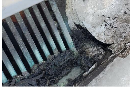
Figure 36. Failed drain flashing at the northmost drain on the west facade.
