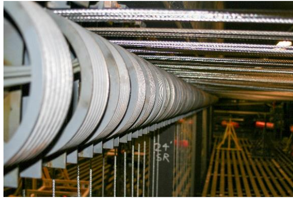
Figure 44. Opera House Rigging
