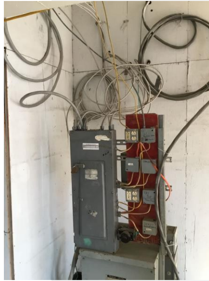
Figure 75. Existing Electrical Panel
