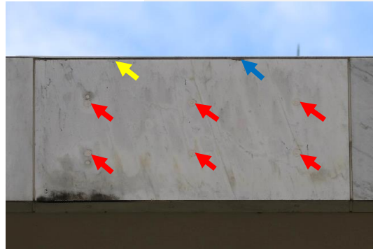
Figure 7. Through-face pins (red arrows), crack (yellow arrow), and spall (blue arrow) at a Plaza Level overhang fascia marble panel (photo taken at the north facade).
