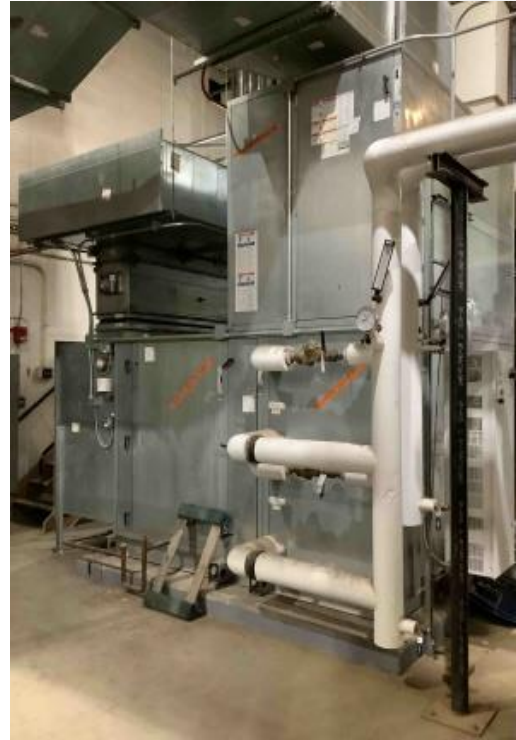
Figure 65. Newer Modular Replacement AHU
