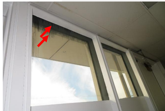
Figure 18. Migration and streaking of the black glazing seals that appears to be on the interior face of both the exterior and interior pane of glass at the Terrace Level (photo taken at the south facade).
