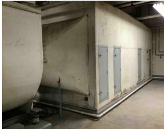
Figure 64. Existing Refurbished AHU – original casing with new interior components
