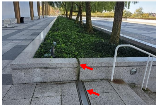
Figure 34. Granite clad planter at the north side of the Plaza Level. Note the expansion joint running through the planter.
