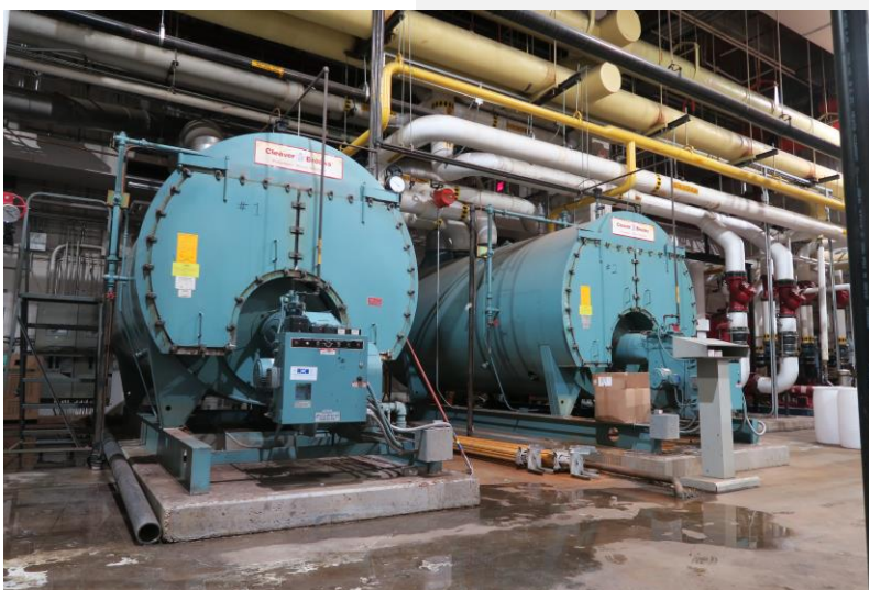
Figure 71. Existing Primary Boilers
