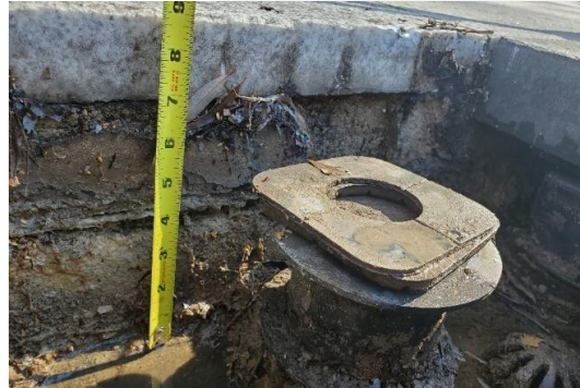
Figure 30. Plaza Level hot-fluid-applied reinforced rubberized asphalt (HRA) membrane and paver assembly at removed paver location.
