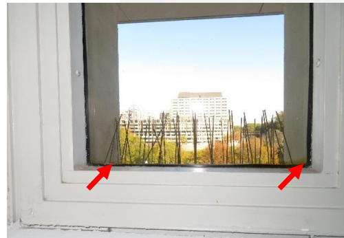
Figure 20. Light bleeding of the exterior black glazing seal material with red-brown staining on the adjacent glass panes.
