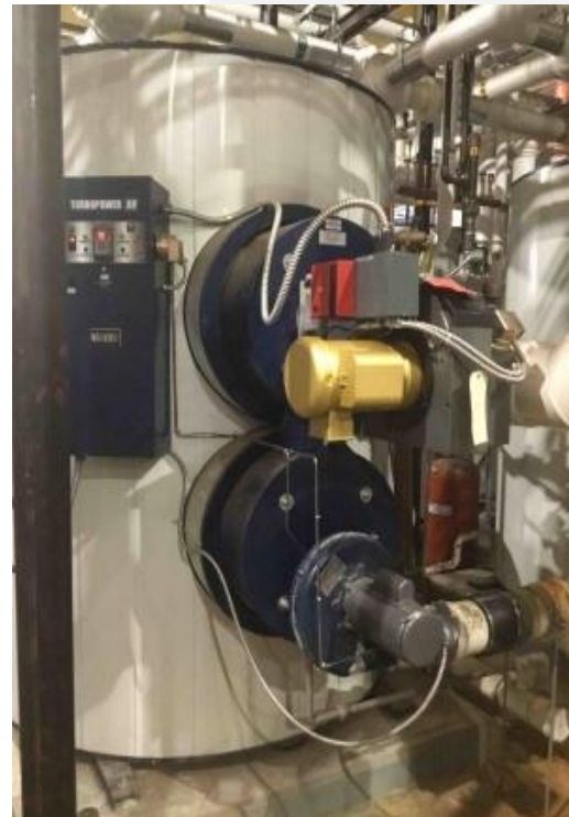
Figure 72. Existing Domestic Water Heater
