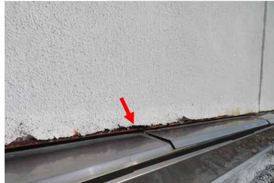
Figure 12. Chipping and corrosion along the stucco panel bottom edge (photo taken at the Penthouse south facade).
