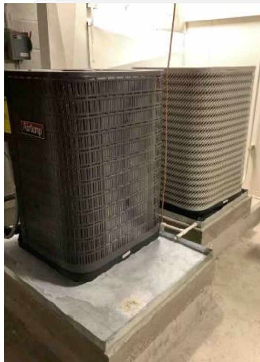
Figure 66. Typical Existing DX Condensing Unit Located in Mechanical Room
