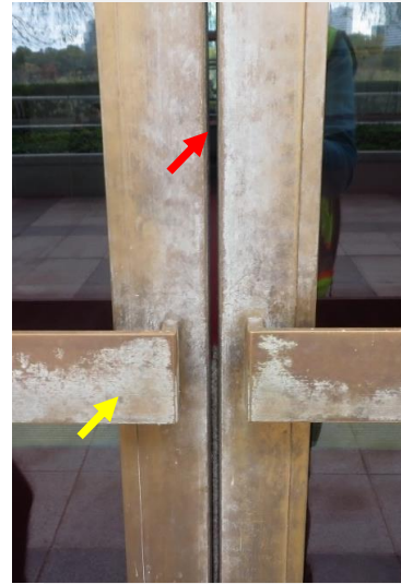
Figure 23. Missing weatherstripping (red arrow) and white-gray discoloration of the bronze surface (yellow arrow).
